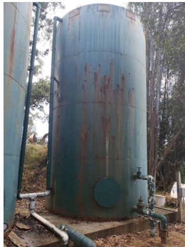
Figure 1 - Existing Tanks in Arrowhead Zone
